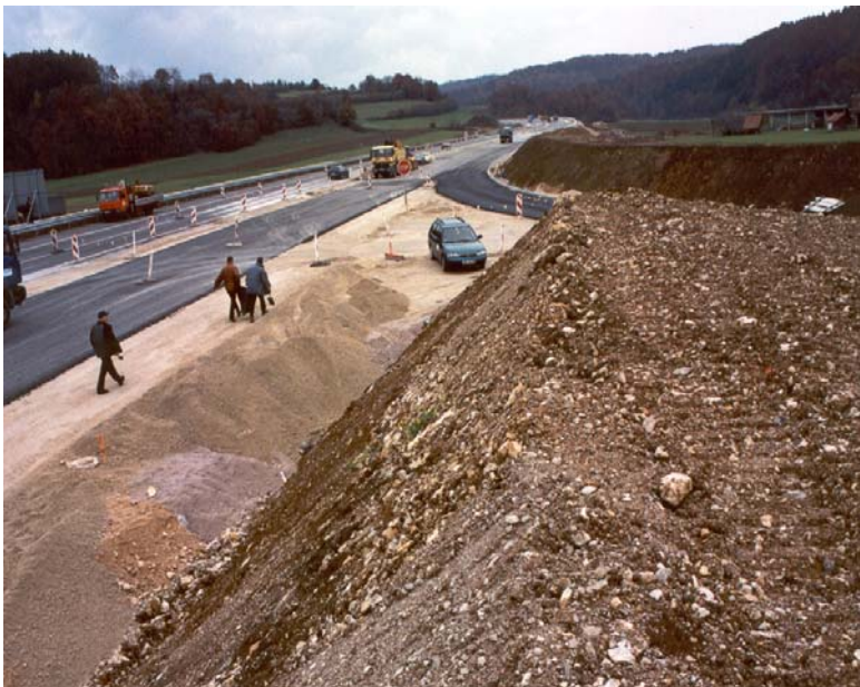
Figure 1.: Artificial composed soil implemented for building the dyke alongside highway Ljubljana – Zagreb (Slovenia - Croatia).
