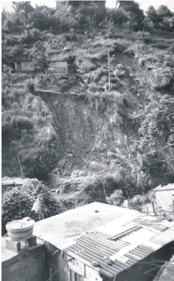
Figure 3.: Taquaril Slope after the landslide occurred on January/2003.
