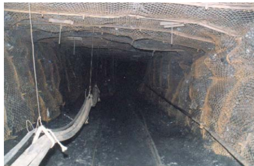
Figure 3.: In-situ support state of roadway along next stable gob (width of pillar, 4m).
