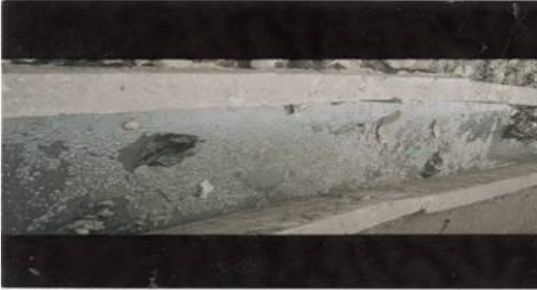
Figure 2.: Drain exposed and blocked with refuse.apart from odour problem, it is a health hazard
